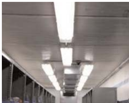
View of interior lighting
