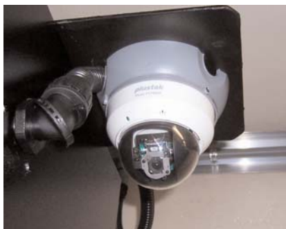
View of surveillance camera mounted on the inside of the portal
